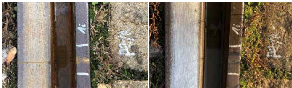
Fig 4. A section of rail surface before (below) and after (right) oscillating rail grinding.
