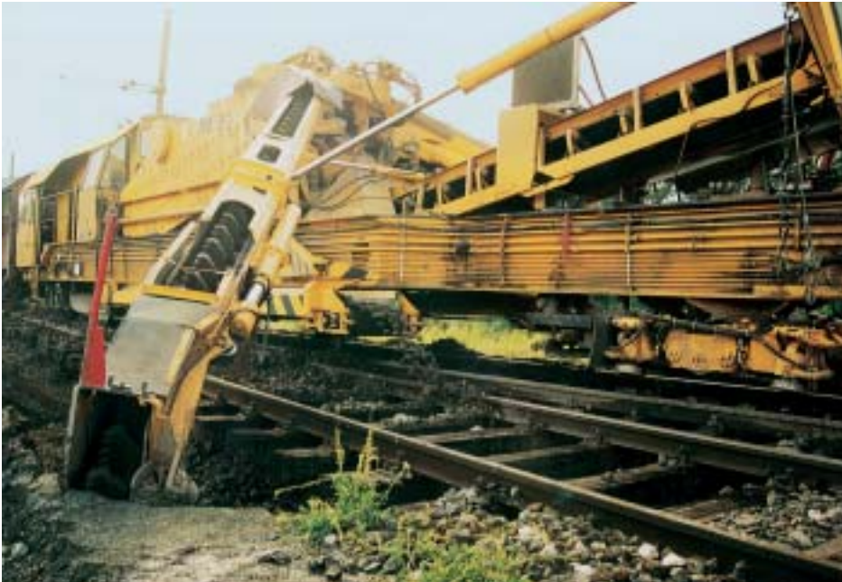
Figure 9: Lengthening the chain cutter bar to extend the excavation width (for cleaning switches)
